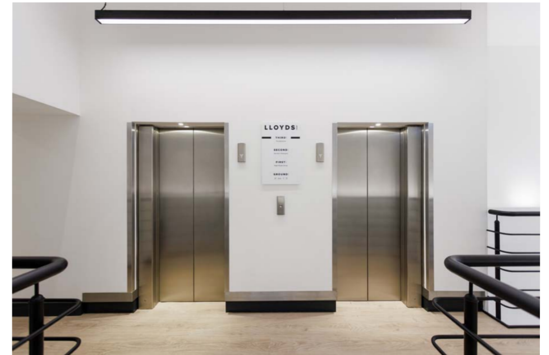
2 X 8 PASSENGER LIFTS
